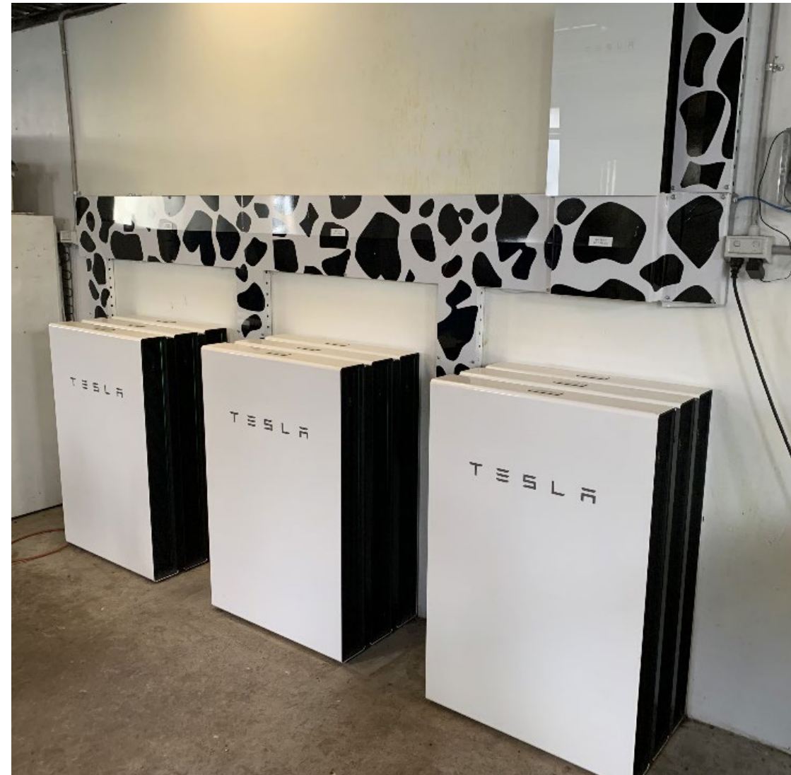
Figure 11: Solar-powered Battery Energy Storage System at Tate's Dairy, Calderwood
