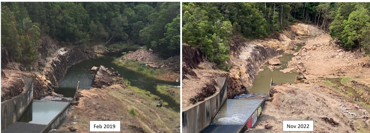
Figure 3 Spillway Erosion Pre and Post Feb 2022 Flood Event
